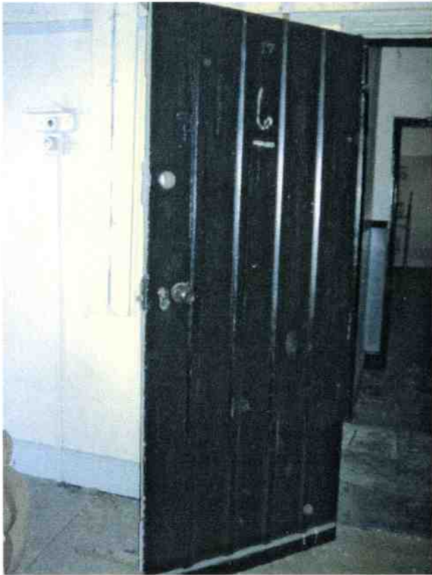
D39 front face, ply sheet and vertical battens over ledged and braced door
