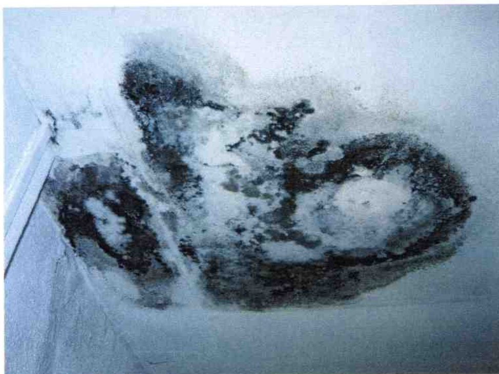
26. S1. Damp staining to ceiling
