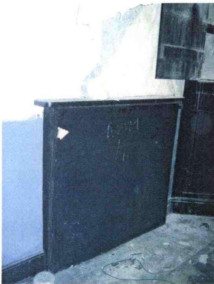
56. S17 Boarded fire place.
