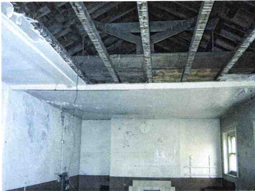
29. S5. Ceiling – damaged by extensive water ingress.
