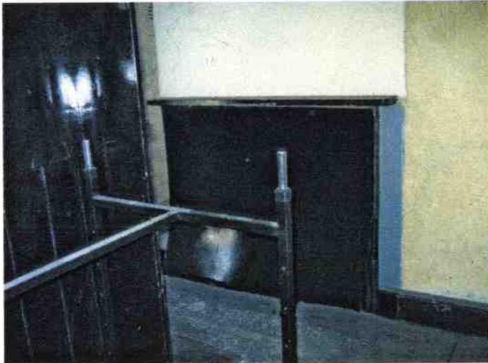
58. S21 Boarded fire place in circulation area adjacent to S12
