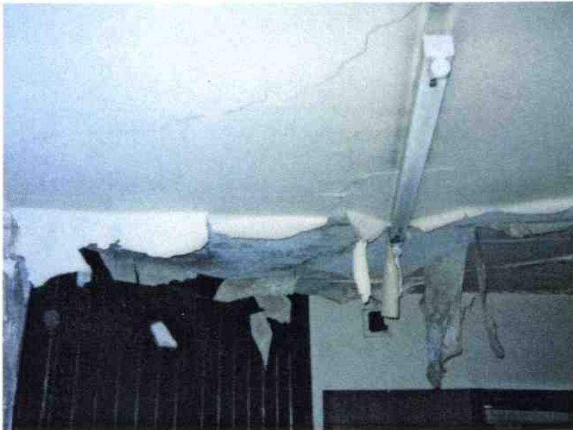
54. S17 Ceiling damage.
