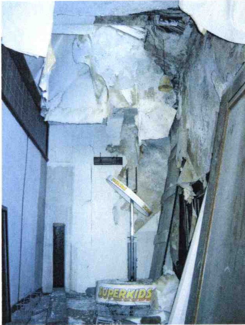
51. S16 rear cubicle area – derelict – severe water damage.
