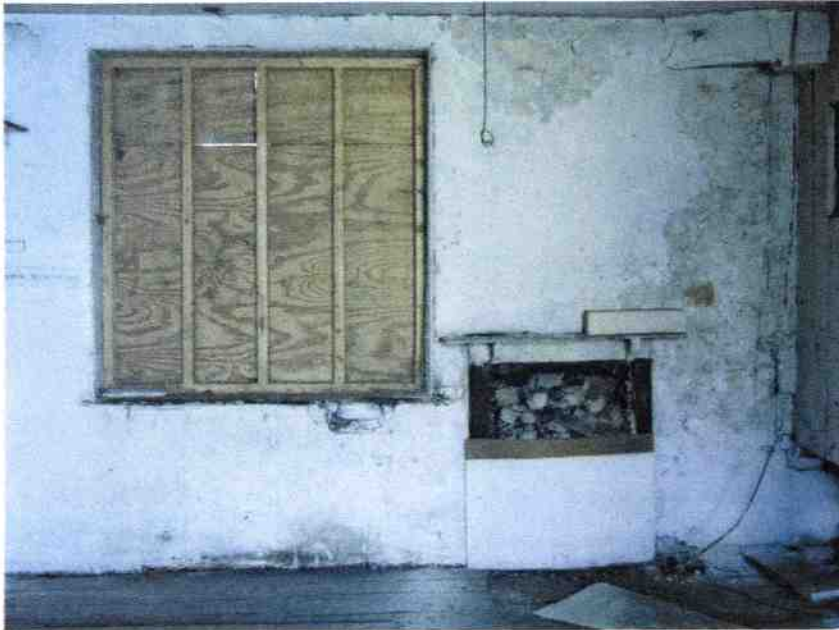
17. W17 – boarded opening. Adjacent fire place opening.
