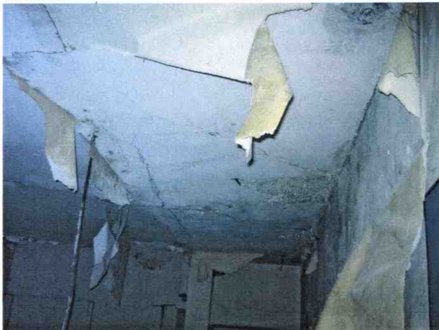
34. S6 Ceiling damage.
